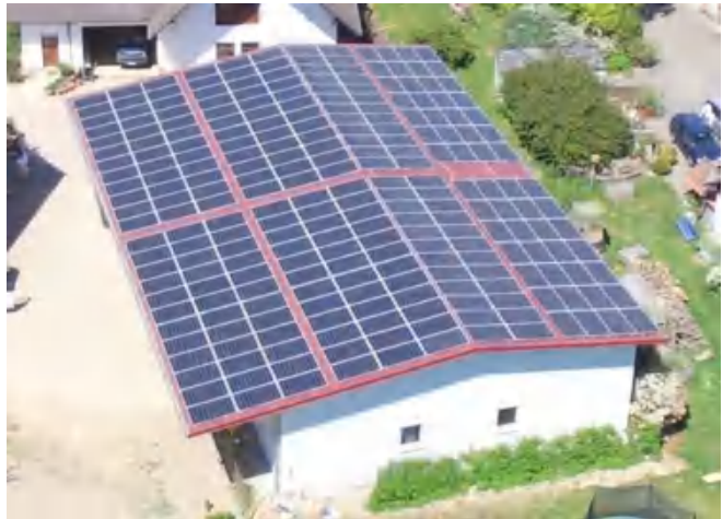
Landw. Halle, 79kWp, 02/20
